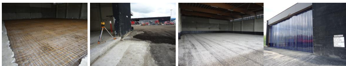
Figure 5 – Reconstruction of a salt storage building after decontamination. The floor is removed and replaced with leak-proof paving - the ground around the storage building is also restructured - a protective coating is applied to the walls inside the storage building - best practice procedures are adopted.
