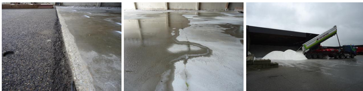
Figure 3 – Indoor salt storage and situations where water and brine can enter the soil
